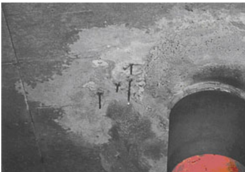
Photo 10: Concrete "icicles" under a bridge on the Tsurumi River (Yokohama City)
