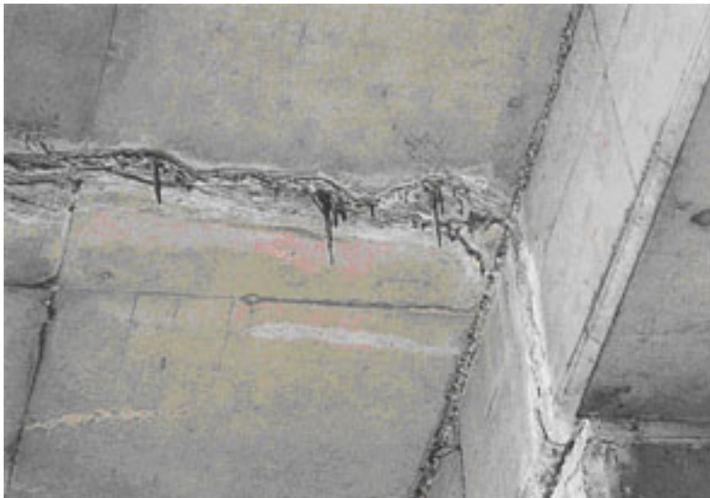
Photo 9: Concrete "icicles" under a highway bridge (Yokohama City)
